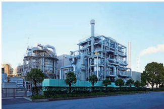
Biomass boiler (Chita Distillery)
