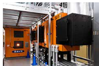
Biomass boiler (Suntory Kita Alps Shinano-no-Mori Water Plant)
