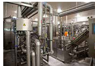
New Air Rinser at our Wiri Factory, Auckland
