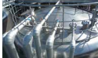
Reuse of water recycled at each stage of cleaning stored in 200 ton tanks
