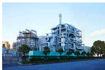
Biomass boiler (Chita Distillery)
