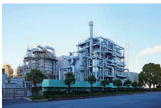
Biomass boiler (Chita Distillery)
