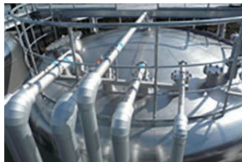
Reuse of water recycled at each stage of cleaning stored in 200-ton tanks
