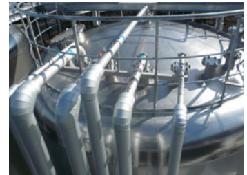
Water is collected according to cleanliness level and stored in 200-ton tanks for recycling
