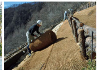
Crumbling slopes are covered with soil and grass rolls, enhancing water-resource nurturing abilities
